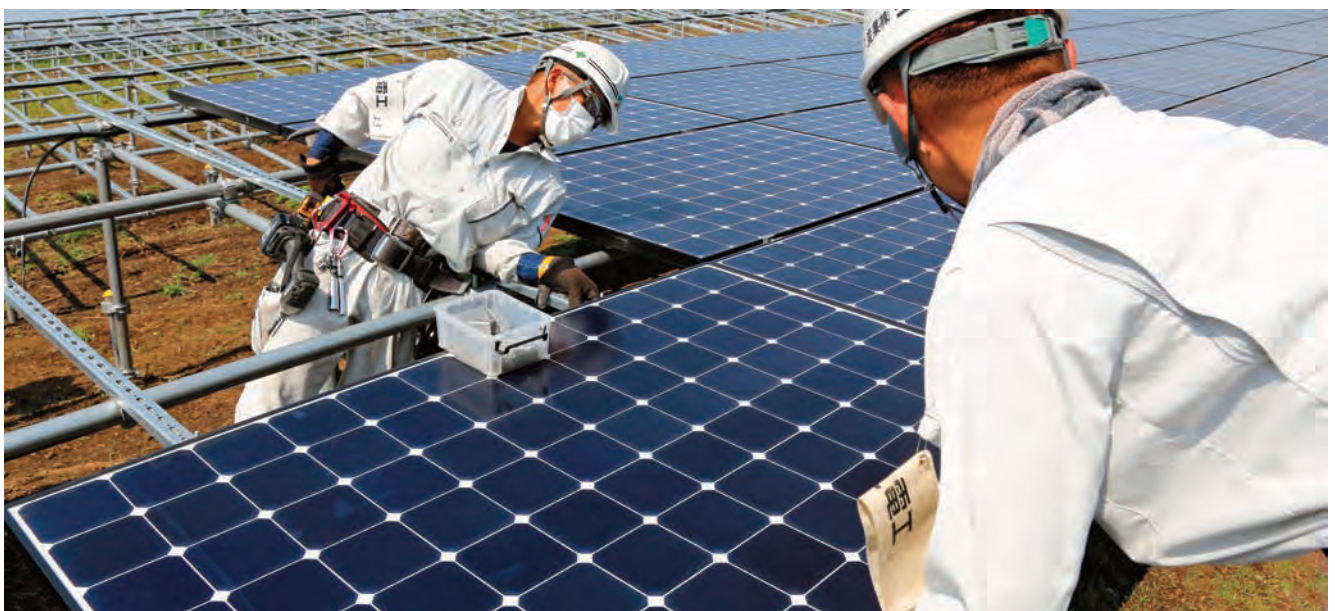
Works for the installation of Sunpower solar panels at Sasyunkan co, Kumamoto, Japan
